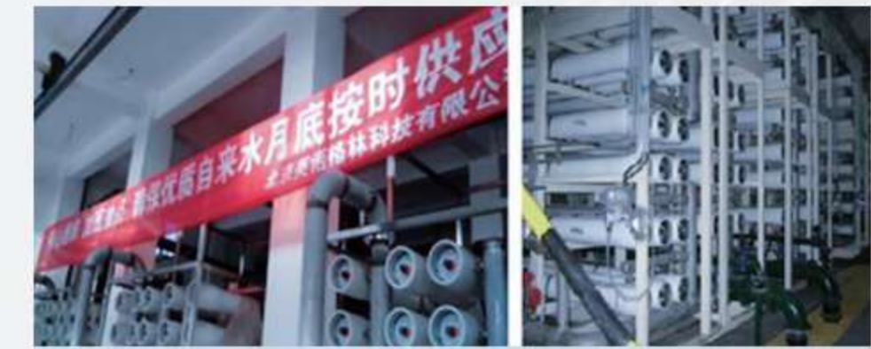
Xilinhot Water Plant, Inner Mongolia Treatment Capacity: 33,600 m 3 /d Main Process: Self-cleaning + Nanofiltration
