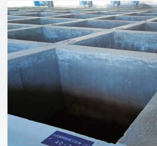
Grid flocculation tank
