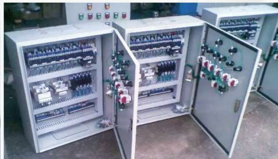
Local operation box
