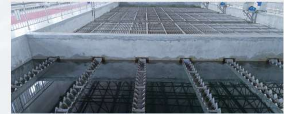
Dongchengfang Surface Water Plant in Zhuozhou, Hebei Treatment Capacity: 150,000 m 3 /d Main Process: Coagulation + Sedimentation + Filtration + Disinfection
