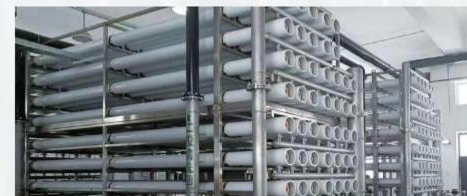
Qiqihar Gannan Town Water Treatment Plant Process Upgrade and Reconstruction Treatment Capacity: 15,000 m 3 /d Main Process: Procurement and Installation of Reverse Osmosis Membrane Treatment Room Equipment + Electrical and Automation Systems
