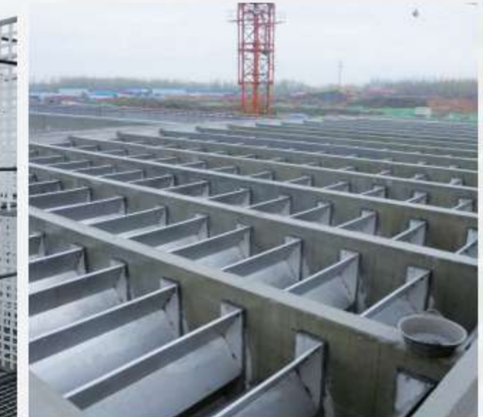
Folded plate flocculation tank
