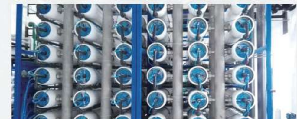
Chaoyang Koubei Water Plant Treatment Capacity: 20,000 m 3 /d Main process: coagulation + sedimentation + filtration + membrane filtration + disinfection
