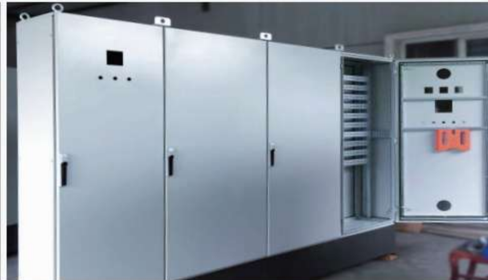
PLC/DCS control system
