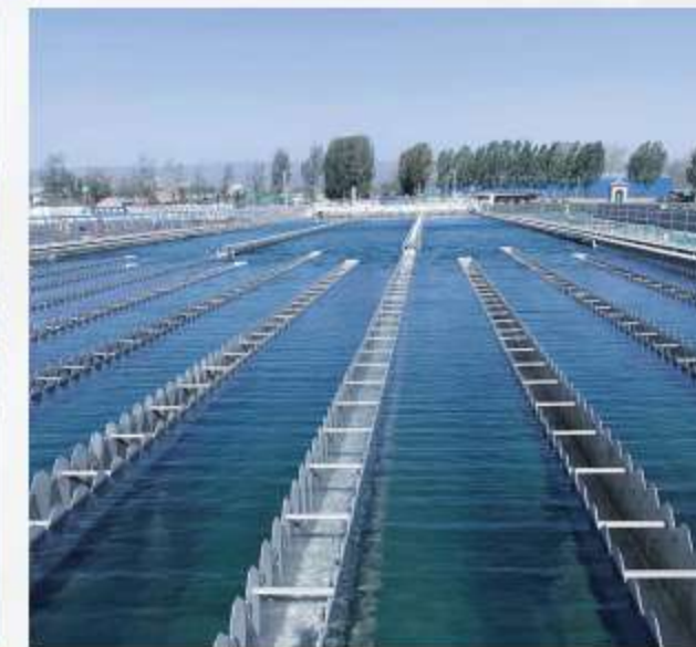
Inclined tube sedimentation tank
