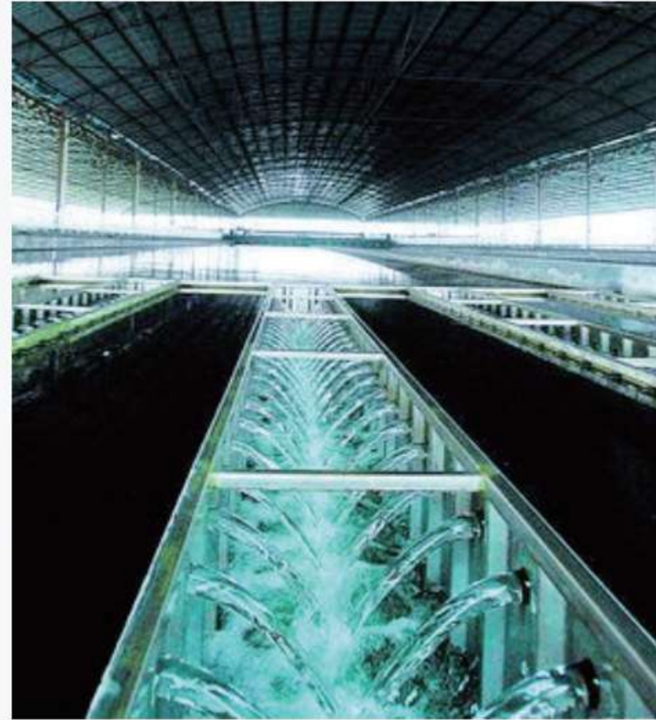
Activated carbon adsorption tank
