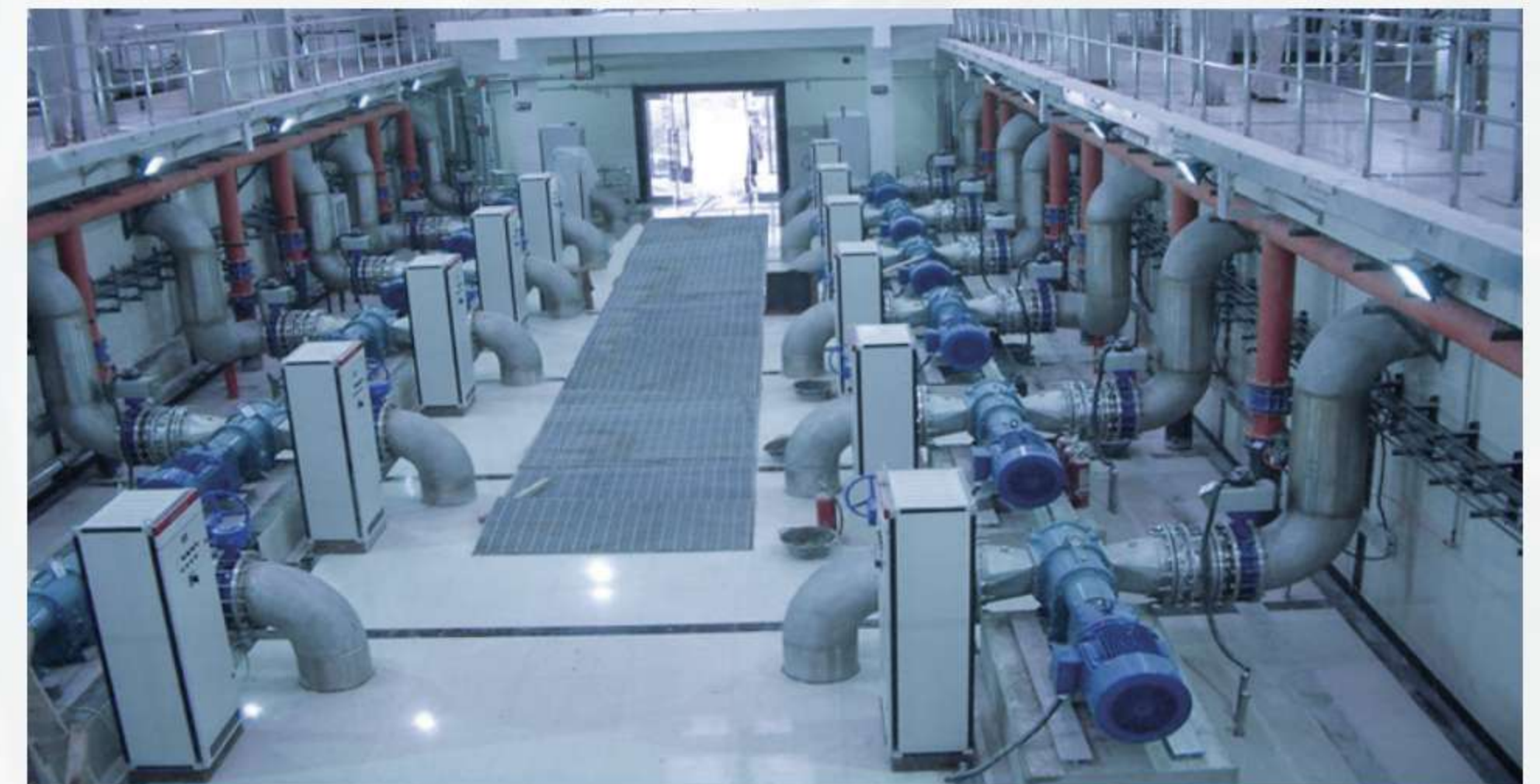
Water pump room
