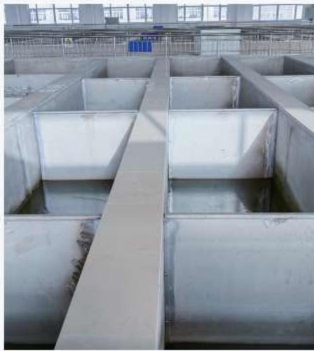
Grid mixing tank
