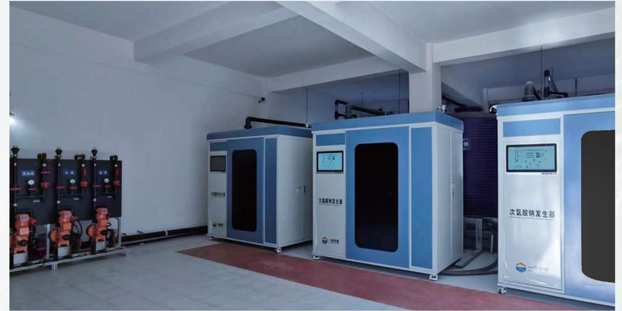
Sodium hypochlorite disinfection equipment
