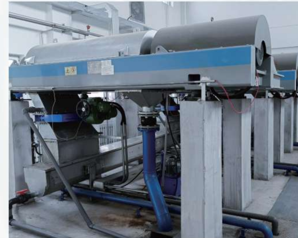
Centrifugal sludge dewatering machine
