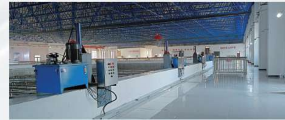
Phase II Project of Rongcheng Surface Water Plant in Xiong'an Treatment Capacity: 25,000 m 3 /d Main Process: Baffle Reaction Tank + Horizontal Sedimentation Tank + Air Flotation Tank + Submerged Ultrafiltration Membrane Tank + Disinfection
