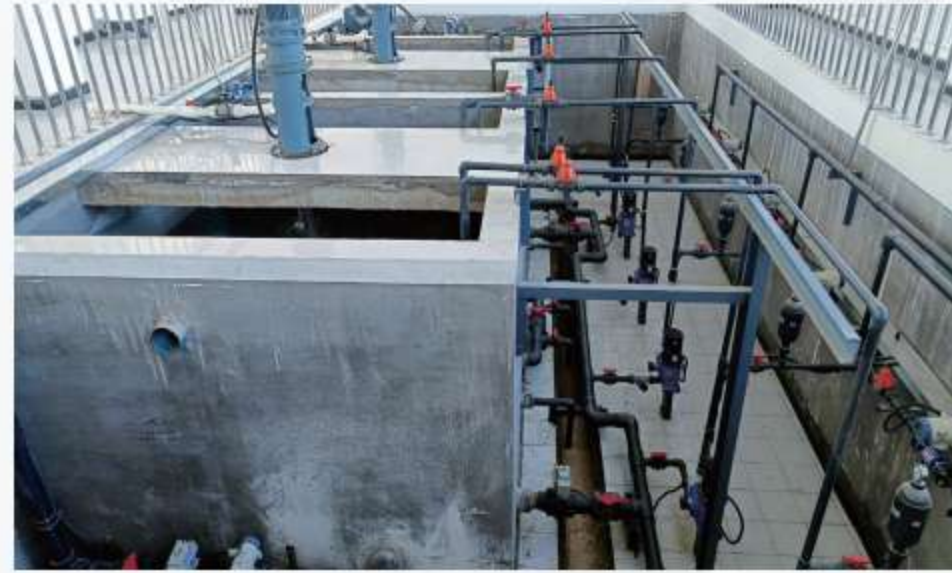
PAC dissolving and dosing system
